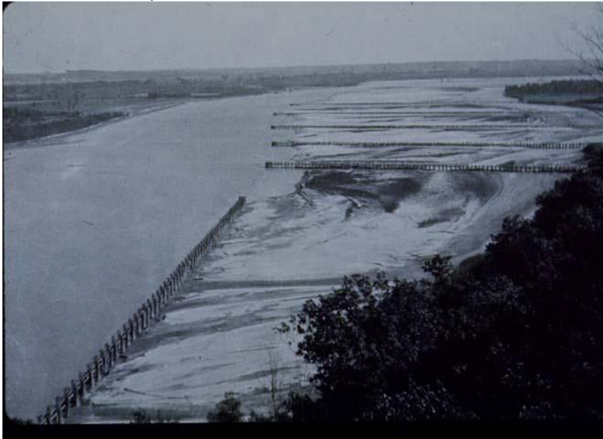
Figure 1: Wing Dikes Construction at Indian Cave Bend, Nebraska, Missouri River, River Mile 517, 10-1935, Source: USACE
